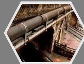
OVER 20,000 MILES OF PIPES
